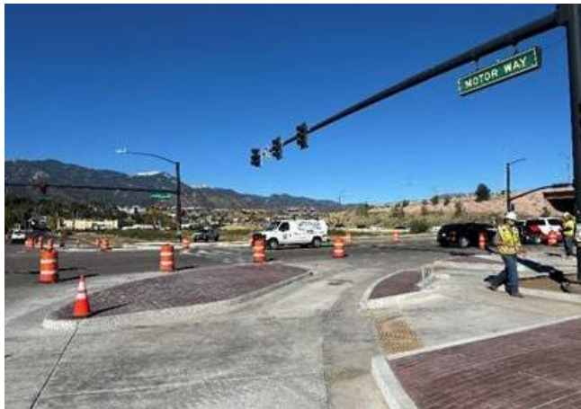
Figure 18. Channelizing islands on Motor Way and Tejon St Intersection, with curb ramps and patterned concrete.
