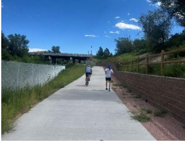
Figure 40. Rock Island Retaining wall and trail construction east of Cascade Underpass. Completed in Fall 2024.
