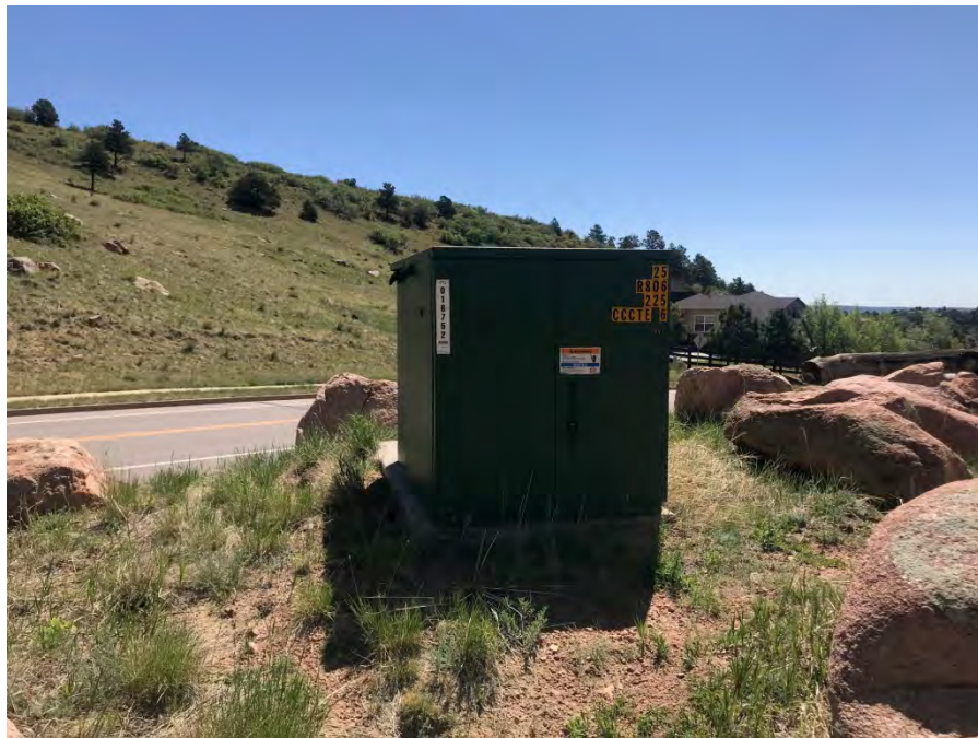
Photograph 2: Pad mounted transformer located on the eastern boundary of the site.
