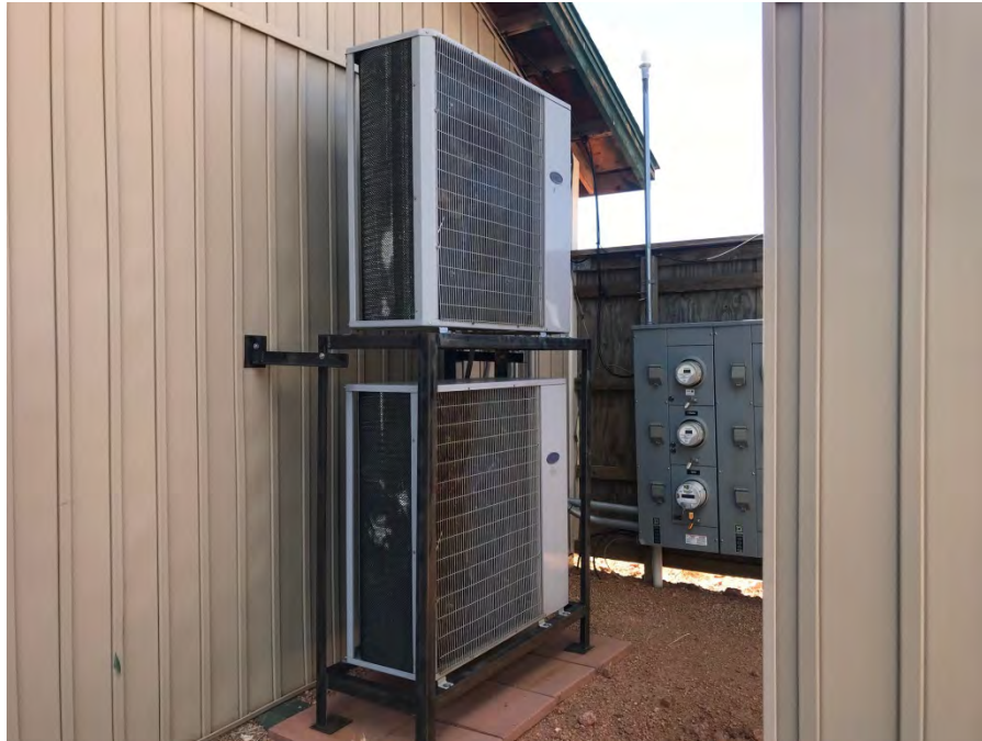
Photograph 21: View of fans and electrical panel located along the west side of the cell tower building.
