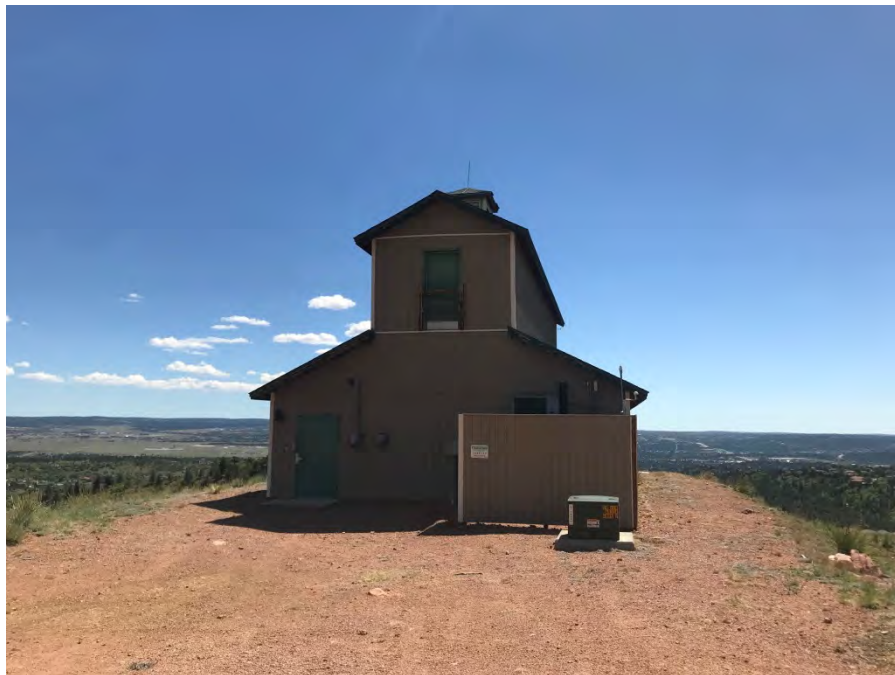
Photograph 20: View of cell tower building and pad-mounted transformer on the central portion of the site.
